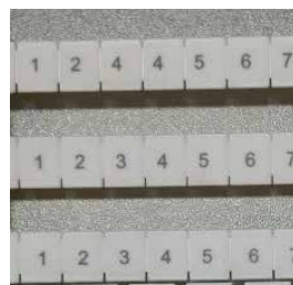
• Electrical mark number identification
